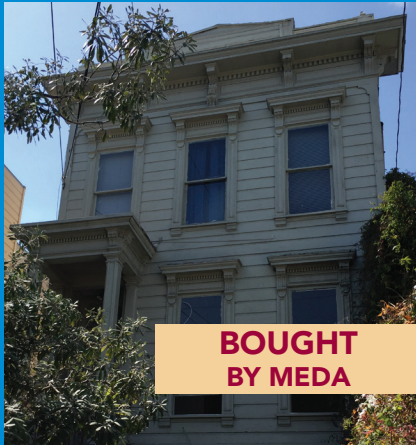
380 San Jose before repairs.
